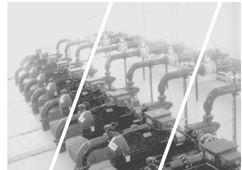
Boosting and Distribution of surface water
