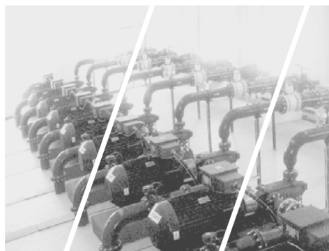
Boosting and Distribution of surface water
