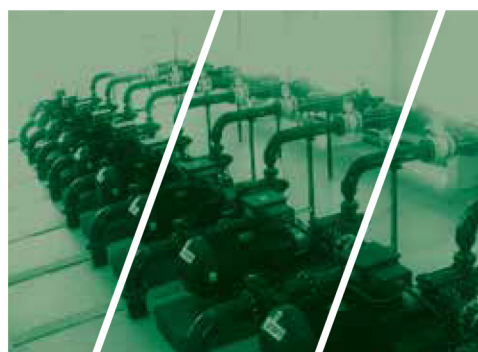
Boosting and Distribution of surface water
